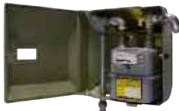
Third stage meter box.
